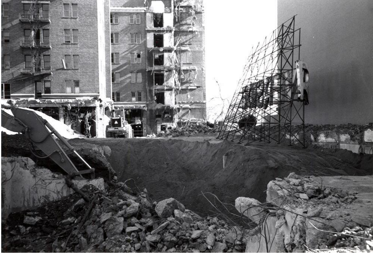
The 1940s-era addition to the Riverside Hotel was removed in the late 1990s when the historic portion was revitalized. Photo by Mella Rothwell Harmon. Image courtesy of Special Collections Department, UNR Libraries.
