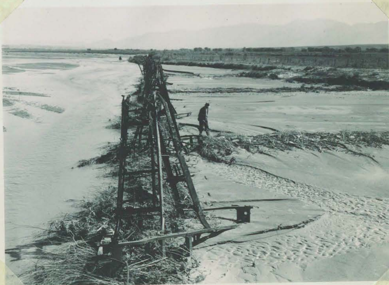
Tetrahedrons prove effective in controlling stream bank erosion. Project developed by Virgin Valley Soil Conservation District in cooperation with the Soil Conservation Service.
