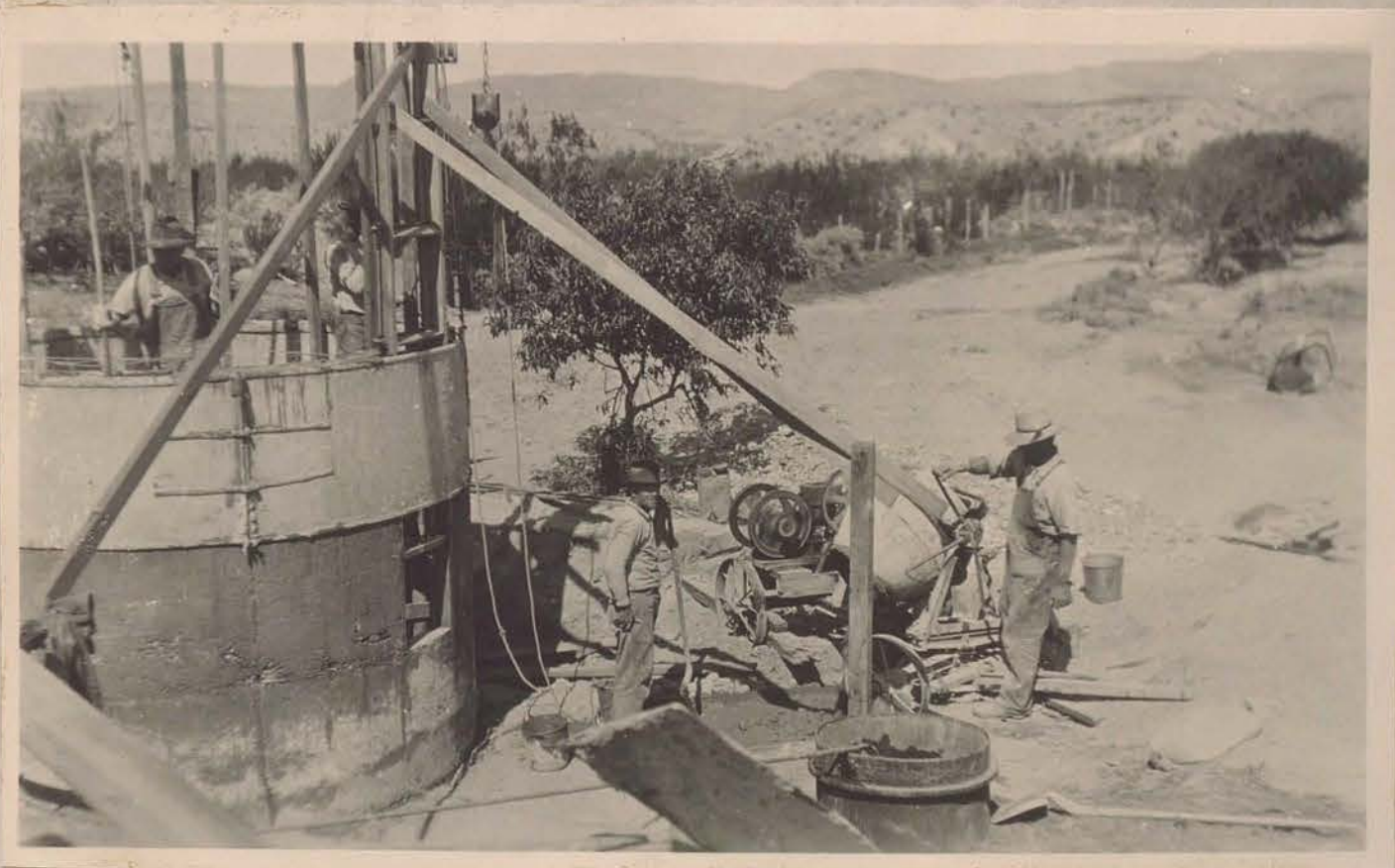
R. C. McKay, Warm Springs, Moapa Valley, in course of construction. Note cement-mixer - Saves about one-fifth time in construction costs.
