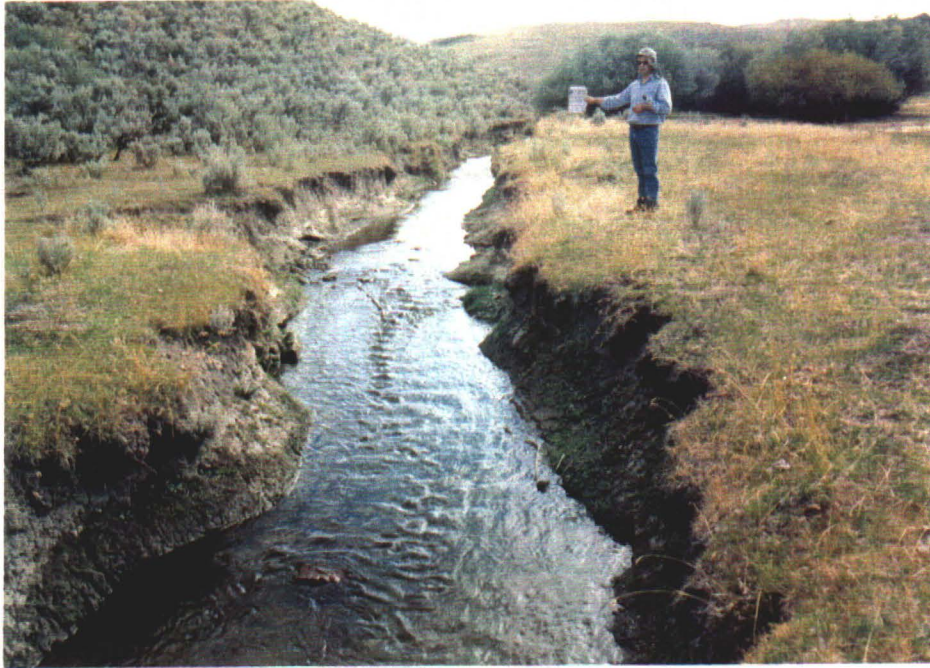
South Fork Little Humboldt River just below the confluence of Sheep Creek. 9-15-98. Although this photograph was taken on private land, poor habitat conditions on public and private lands upstream have led to accelerated channel entrenchment and associated baselevel lowering of the entire South Fork of the Little Humboldt system in the Little Humboldt Allotment.
