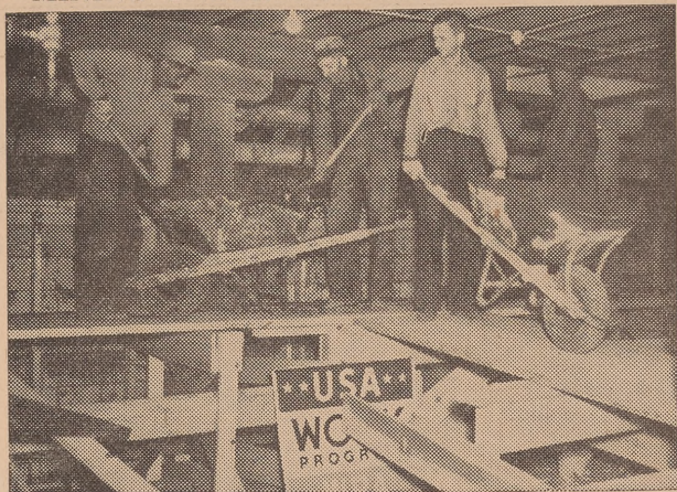
With excavation work already completed, WPA workers pour concrete for the walls and floor of the new basement beneath the Mackay School of Mines building.
