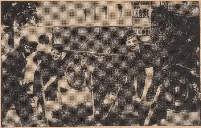
Coeds work too—in clearing bricks and building roads in Warsaw so their city may live again. WSSF is the main Polish source of food, clothing, medical care, and housing for many of these students.
