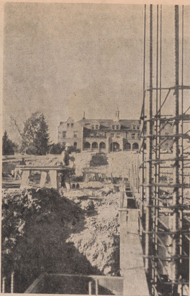
THIS IS the construction site of the Jot Travis Memorial new Student Union building on the north shore of Manzanita Lake. The Student Union will house all the student body offices and an ample recreation area.
