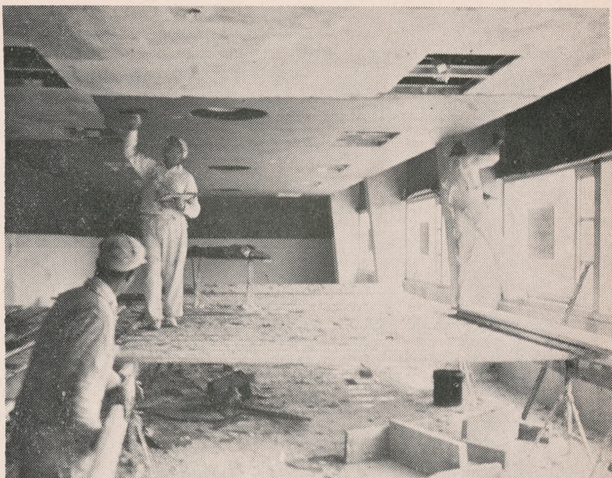
WORKMEN RUSHING to complete the new Jot Travis Student Union building before the Spring semester closes. The building had to be cut in size due to lack of funds. Already too small, space may still be cut by moving in the ASUN book store (Plastered Photo)
