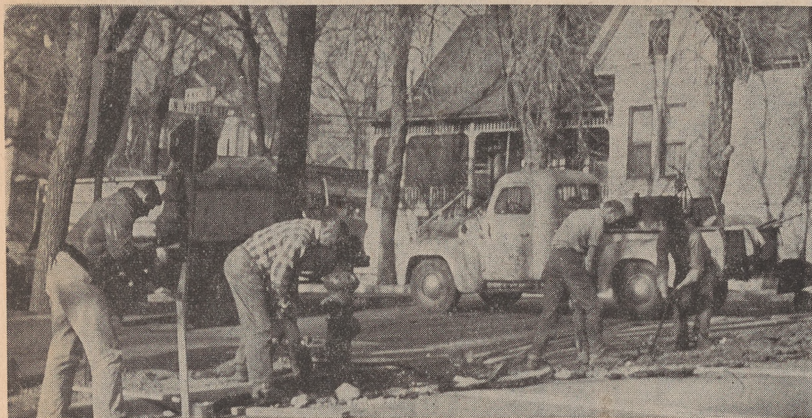
THE LONG-AWAITED Ninth and Virginia traffic signal system is now being installed. Men have been laying the groudwork for the signal poles for the past two days. Workers in this picture are digging a trench across Ninth street. Several weeks ago, a petition calling for installation of signals here was signed by University students and sent to highway officials. The petition was prompted when a woman was killed at this corner recently.
