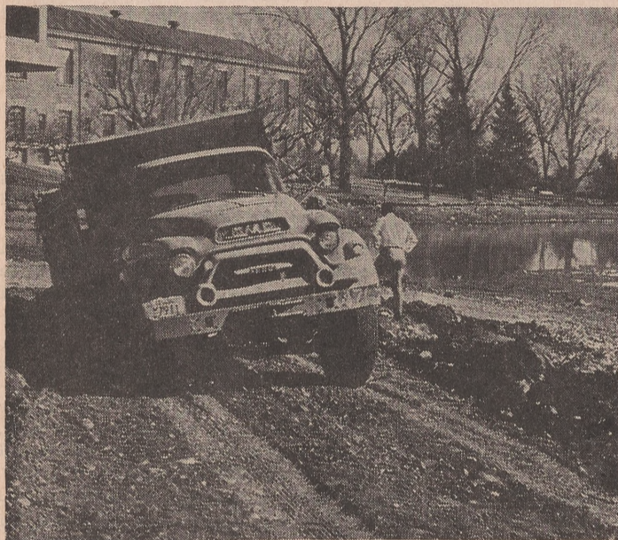
TRUCKS HAUL debris from Manzanita Lake's bottom in Blue Key's "Operation Mud." (See related story on Page 3.)
