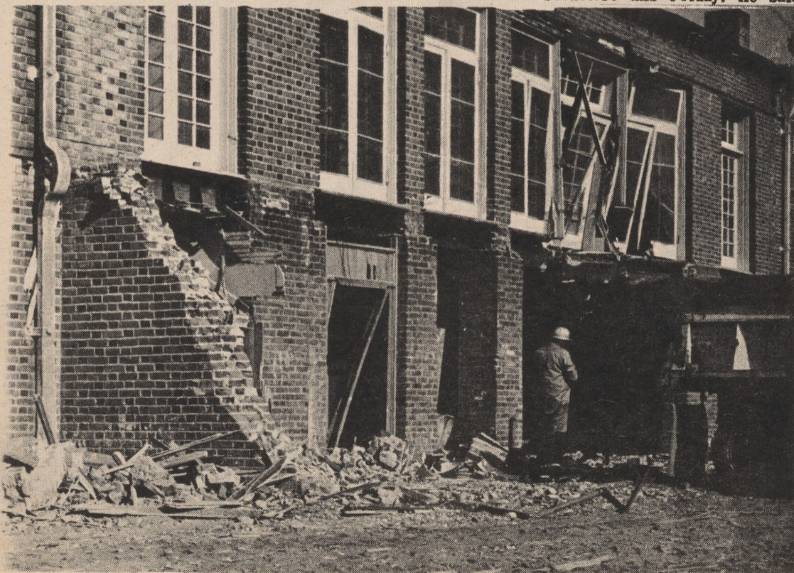
The picture shows the last days of the 'old Mackay Stadium' field house. Here the football teams of the past would come to begin their games, and leave to begin their celebrations, or decide how to do it better next time. The field house is being torn down to make room for the new physical sciences building.
