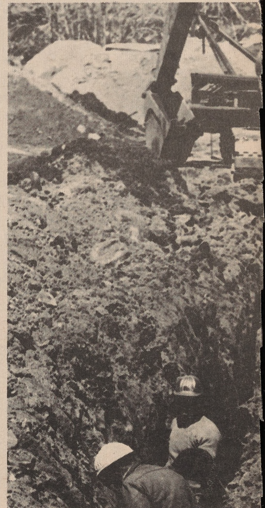
Construction crews are now coming down from Incline Village with an 8-inch sewage line which will carry over
