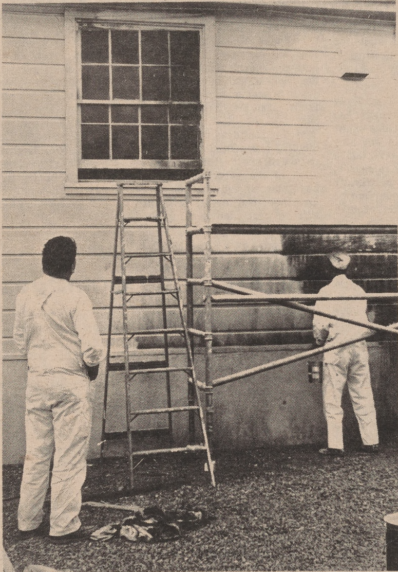
Workmen spent the day at Hartman Hall trying to repair the damage done by an unknown firebomber yesterday morning. (Photo by Dan Smith)
