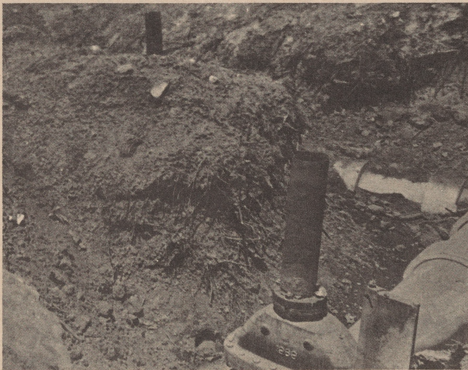
Progress protrudes in the form of an exposed sewage line. This is only one section of an entire network of lines which are inevitable with the coming of suburbia to Lake Tahoe.
