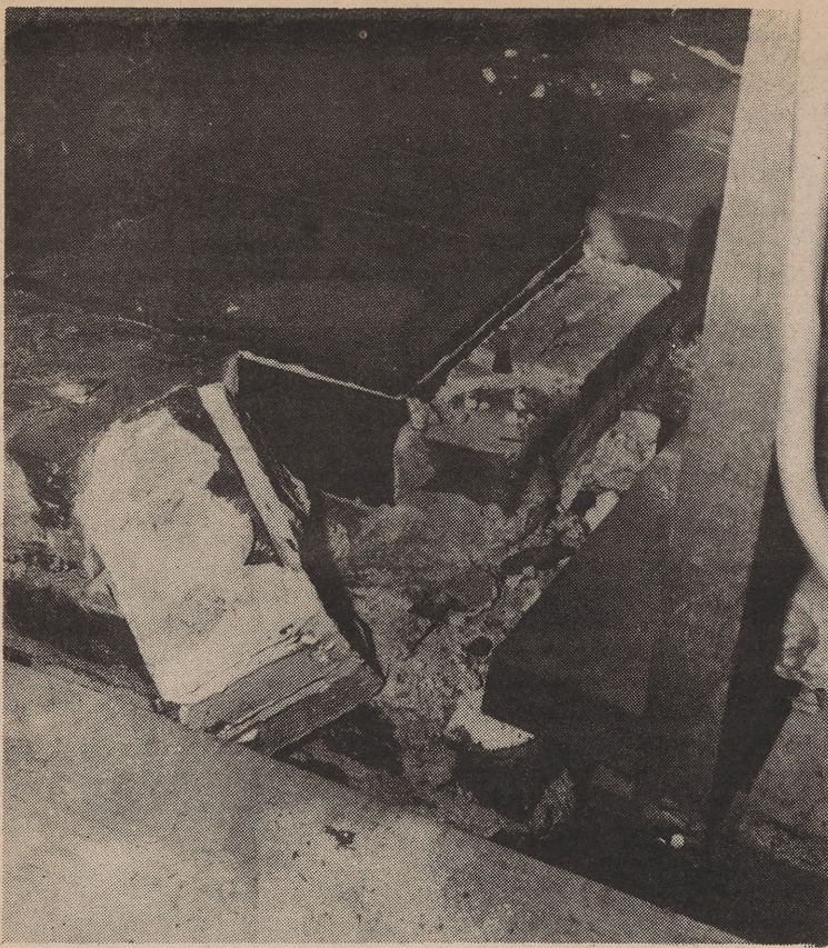
The top story of the Electrical Engineering Building is crumbling down.
