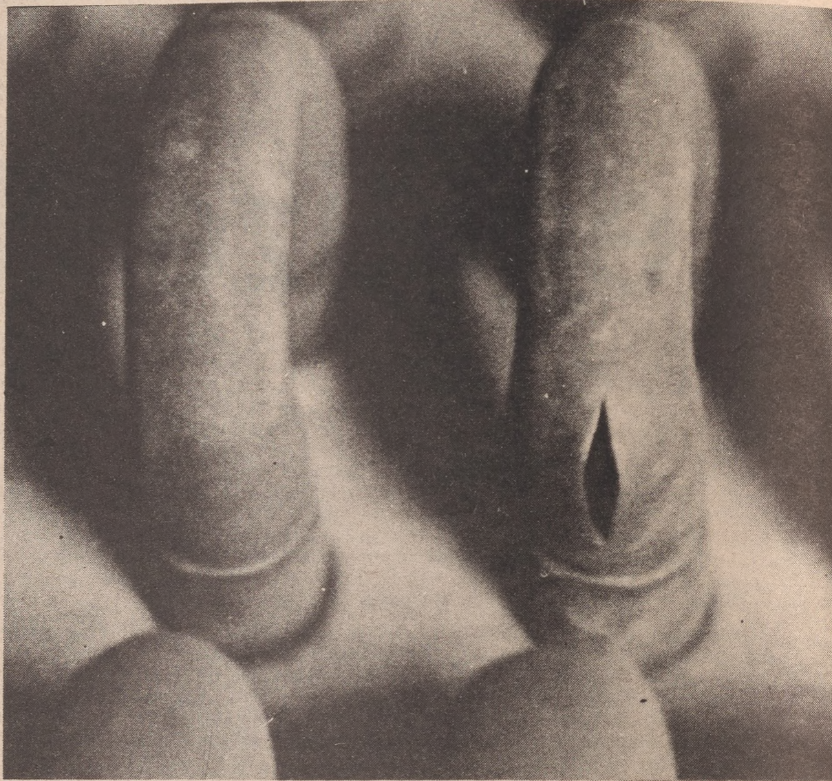
This is an example of the many ruptures in the copper tubing of the air conditioning unit for the chemistry building which burst due to freezing.
