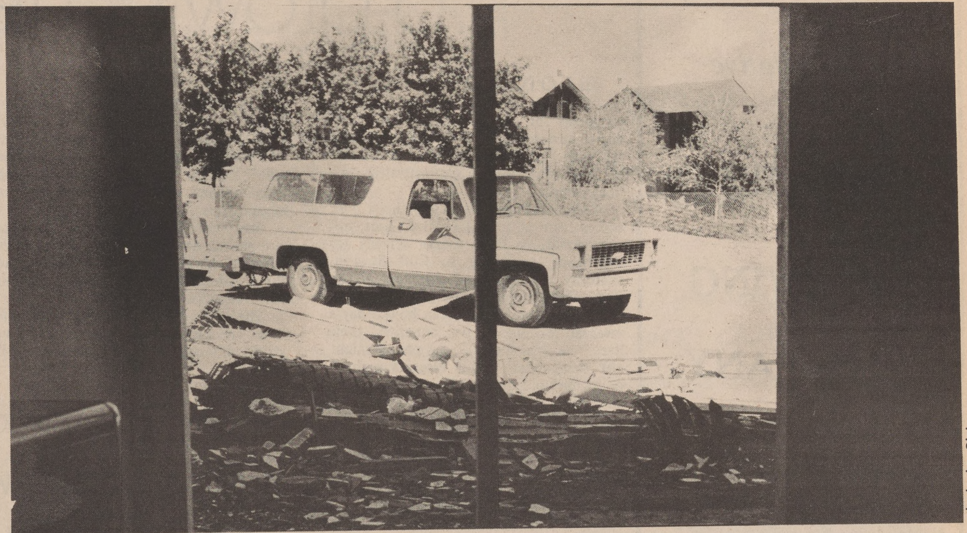
Student union expansion, to be completed next fall, is still in demolition stage, as shown in open-air view from the ASUN office.
