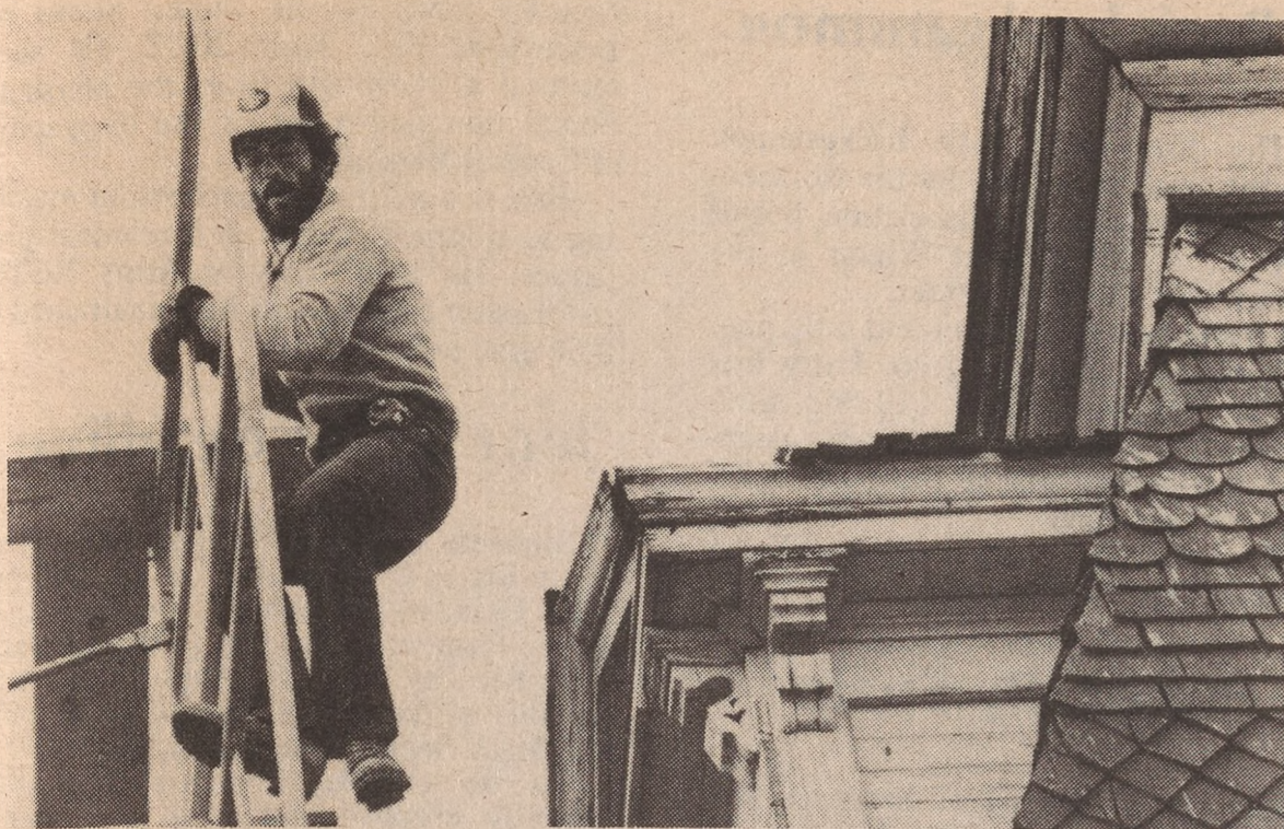
Hard hats are on, chain-link fences are up and equipment is rolling in at the south end of the quadrangle. The long-awaited restoration of Morrill Hall has begun.
